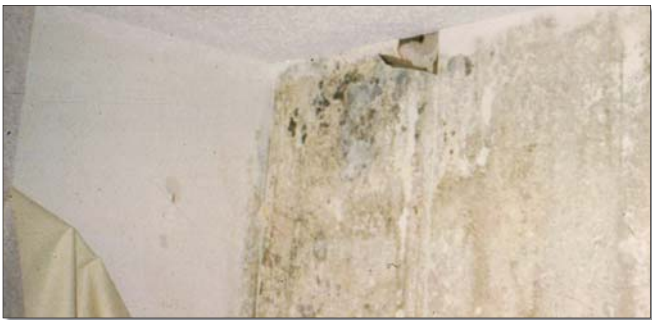
Photograph 4: Hotel Room Flow Path. Mold on interior wall resulting from exterior humid air being pulled into demising wall as a result of negative pressure field created by leakage of exhaust fan in bathroom dropped ceiling.
